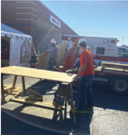
Janotta & Herner spent a Saturday building floors for the tents set up to handle a possible influx of patients due to COVID-19.
